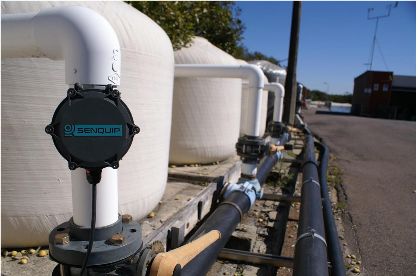
Figure 2 - Battery Powered ORB-X1 Monitoring Filter Pressure
